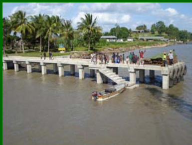
Sturt Island jetty recently constructed and open to the public (Picture from Nawae Construction Ltd)
