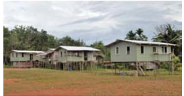
Some of the 35 houses being built at Gresohore village. This project is being funded through the Tutuwe Trust
